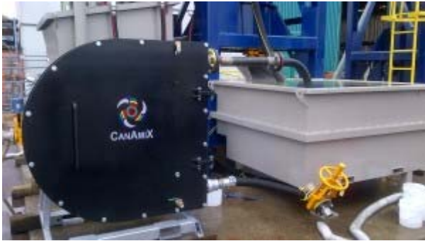
A 100mm pump on Fine Grinding Mill
