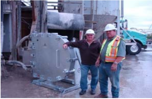
A 100mm pump on cement transfer
